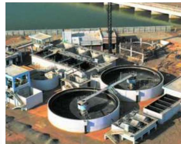
Sewerage Treatment Plant 10 MLD Commissioned, expandable upto 30 MLD
